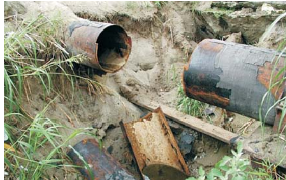
Damaged section in the pipeline from NIS Oil Refinery to HIP Petrohemija Pancevo, September 2002
