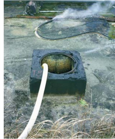
Oil stains on soil and manhole at NIS Oil Refinery, Novi Sad
