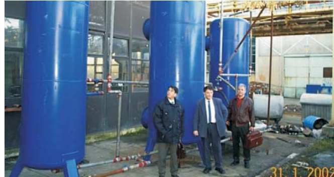
Device for treatment of PCB-contaminated wastewater from paint hall pits, January 2002
