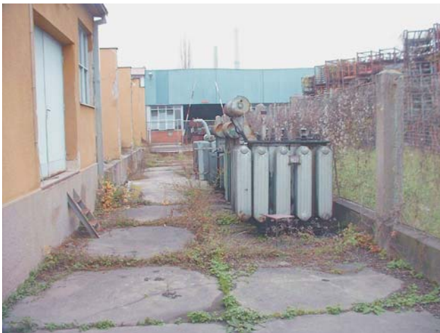
Storage of PCB contaminated equipment, Zastava
