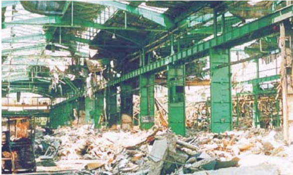
"Zastava" paint hall after bombing, June 1999
