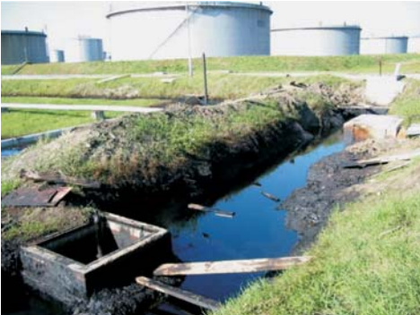
Malfunctions in sewerage system at NIS Oil Refinery, November 2002
