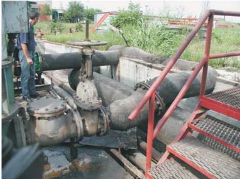
Beginning of the pipeline from NIS Oil Refinery to HIP Petrohemija Pancevo, September 2002
