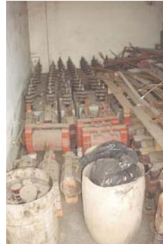
PCB containing capacitors stored at the site, removed and disposed, December 2003
