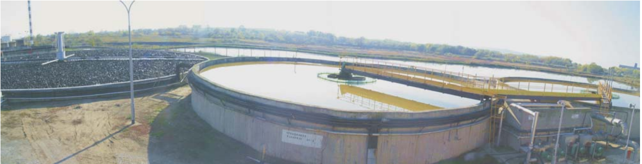
HIP Petrohemija wastewater treatment plant (bio-filter, secondary clarifier - front), and unlined sludge lagoon (behind)
